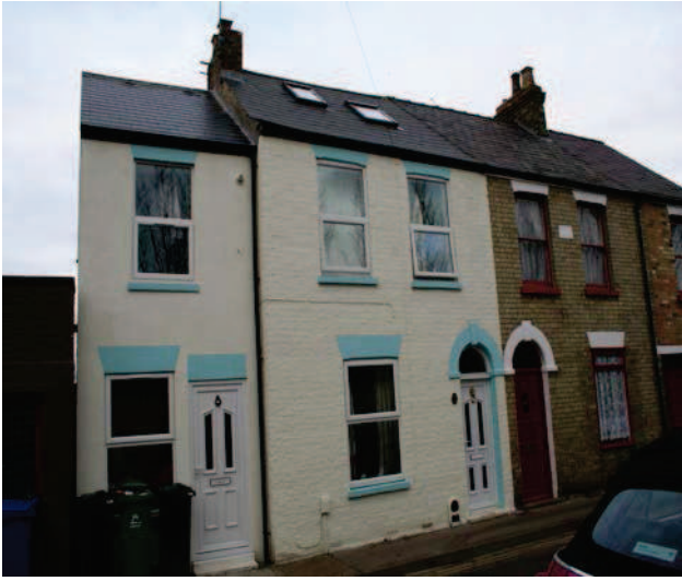
Poor replacement doors
